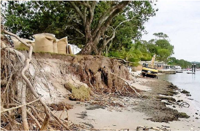
Coastal erosion before the project began
