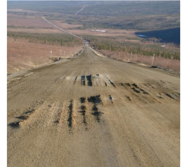
Basecourse rutting due to thaw weakened subgrade
