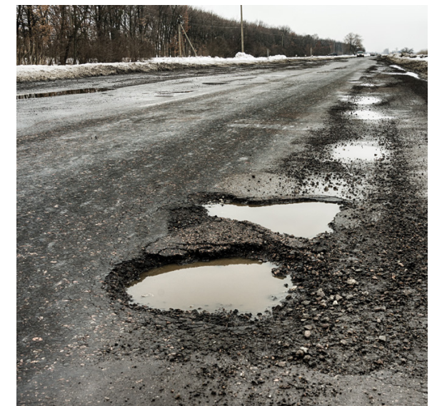
Frost boil through cracked pavement surface
