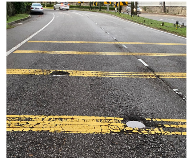
Potholes formed due to spot weakening of the subgrade
