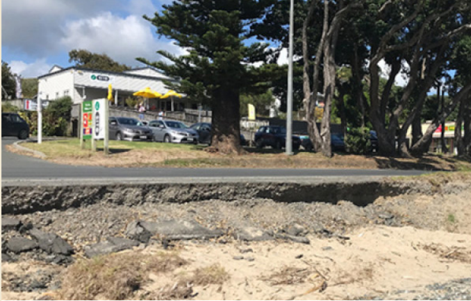
Road erosion before project commencement.
