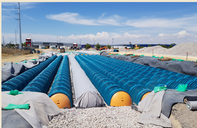
The design consists of five separate tanks across the site catering for approximately 1547m 3 of stormwater storage.
