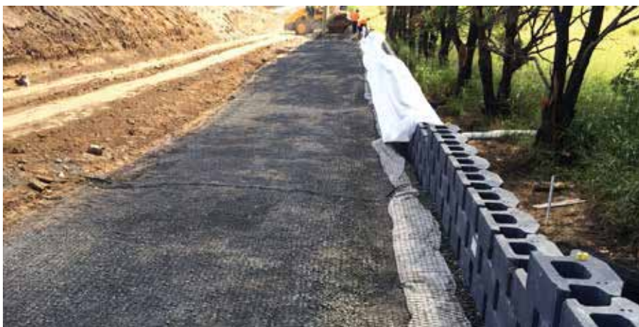
Construction of the reinforced segmental block wall using Miragrid® 8XT geogrid reinforcement cut to design length
