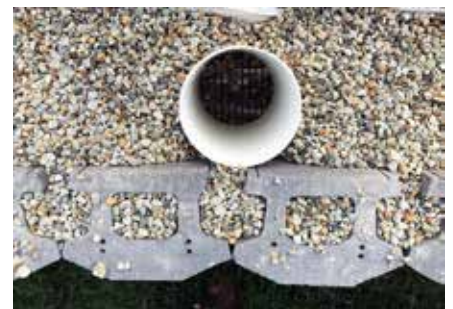
View of PVC pipe immediately behind block facing to house outer guard rail
